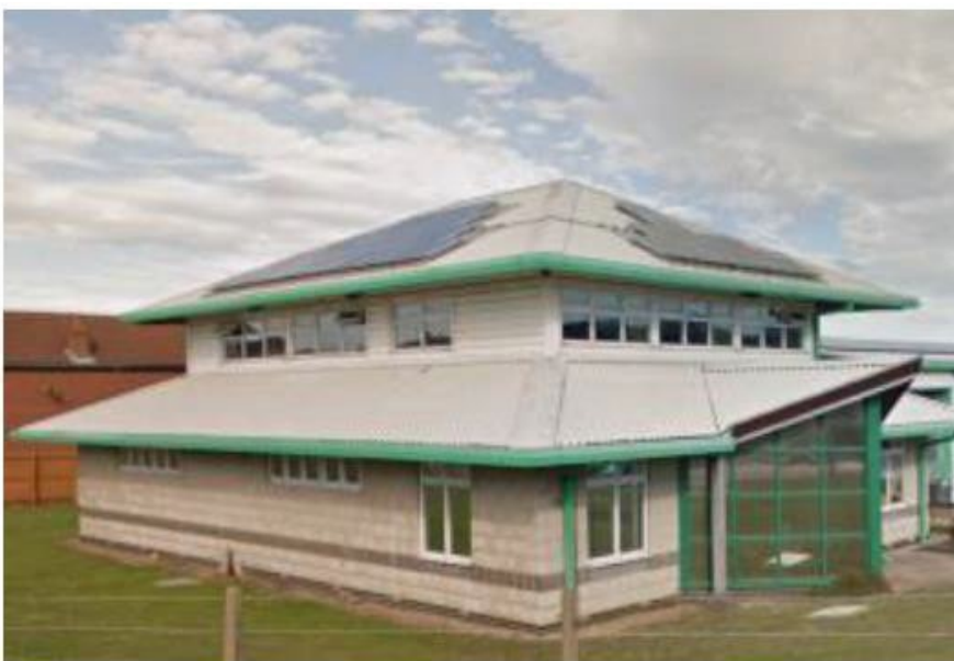
Solar PV installations on EEAST site
